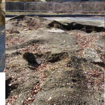
Sink holes from failed culvert
